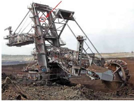
Fig. 3 Bucket wheel excavator SchRs630, gusset plate crack position [3]
